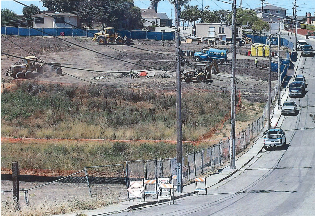
Heavy equipment is shown working the land for a new housing project on the 100 block on Miles Lane in Watsonville. — Tarmo Hannula/The Pajaronian
