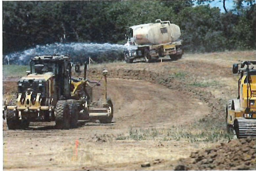
Heavy equipment shapes the land between Brewington Avenue and Atkinson Lane at the start of a new housing project — Tarmo Hannula/The Pajaronian
